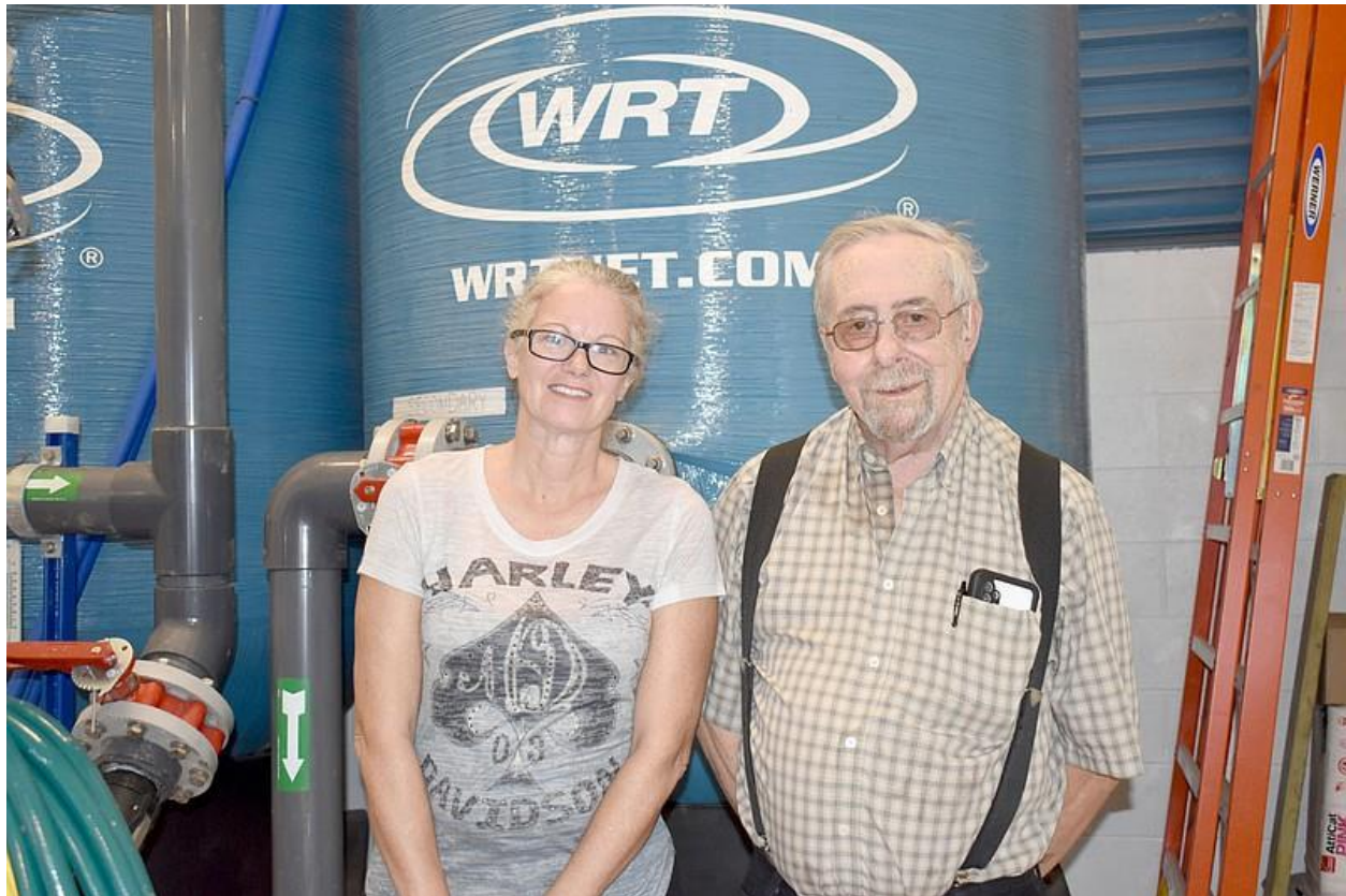
Lanagan Mayor Pro Tem Teresa Ezell, left, and Lanagan Mayor Stan Haywood are pictured in front of the radionuclide tanks at the new water treatment plant.
