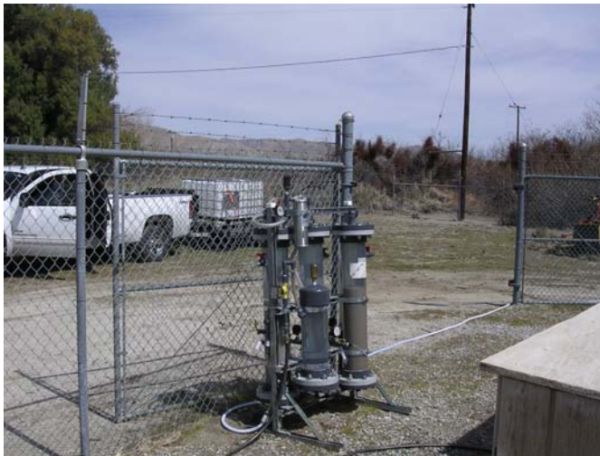
Typical Z-92 ® 3-Column Pilot Test Equipment.
